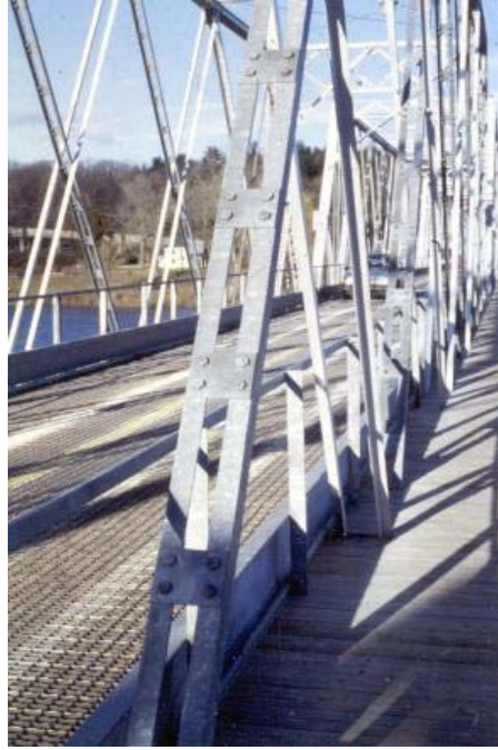
Figure 3. Detail of Delaware River Bridge at Washington Crossing, NJ. Undersized and deteriorated truss members of the 1904 bridge were replaced in kind with higher strength steel to increase the load carrying capacity. Note that the new built up members have high-strength bolts instead of the original rivets. The wood deck was replaced with an open steel grid deck, which also increased load capacity. Photograph by Lichtenstein Consulting Engineers, Inc.
